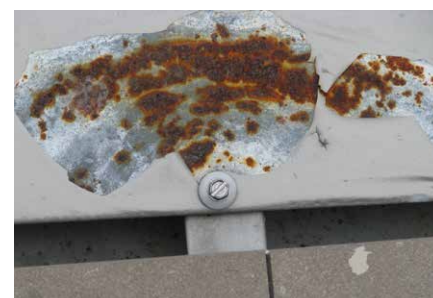
When the paint is removed corrosion down to base steel is clearly visible.
