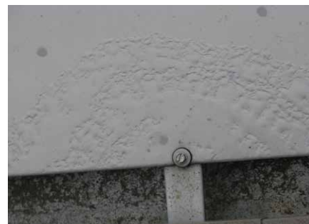
Paint bubbling radiating out from stainless steel fastener on roof 300ft from ocean.
